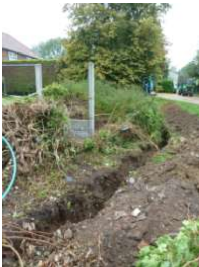
Location of the Water Meter
