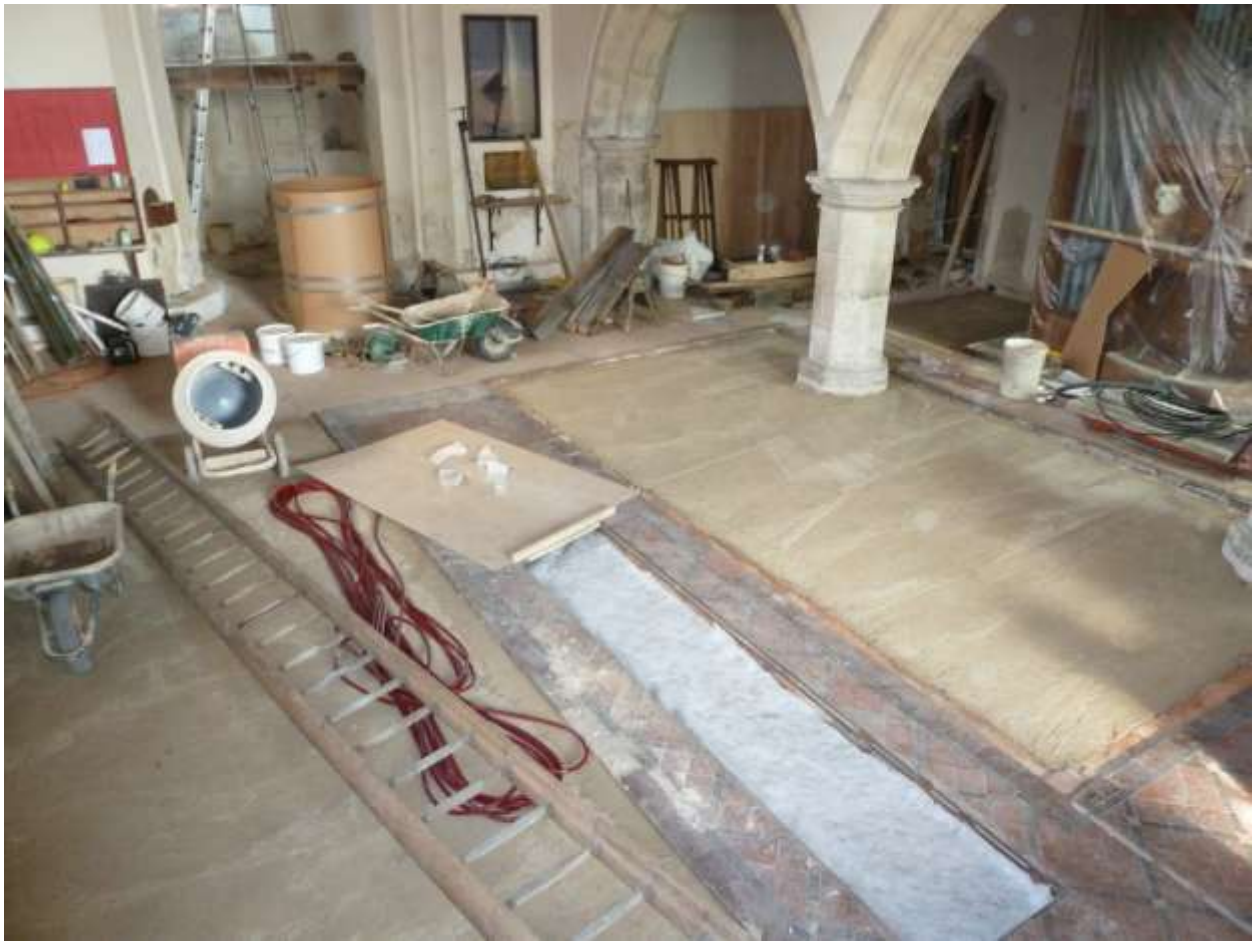
The nave and north aisle floors filled and leveled ready to receive the final screed and tiles
