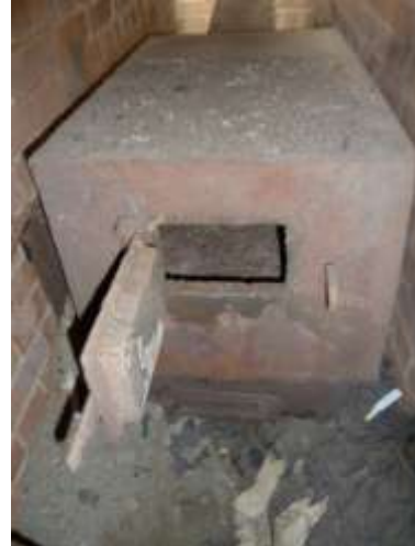
Boiler with coke still inside
