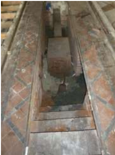
Victorian coke burning boiler Located under the Aisle of nave
